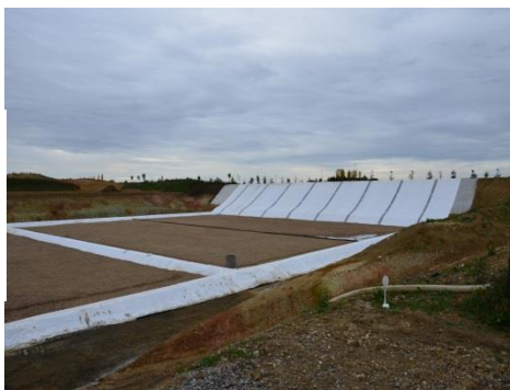
Solid waste management Loches – France – Production of Biogas Source: Naldeo 2015
