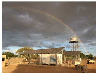
Solar powered brackish water treatment unit OSMOSUN® for community water production in Mozambique
